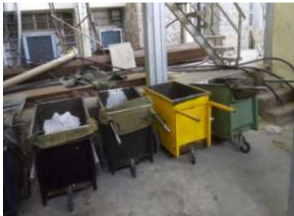
Fig. 4.12: Open parking for waste trolleys without lids
