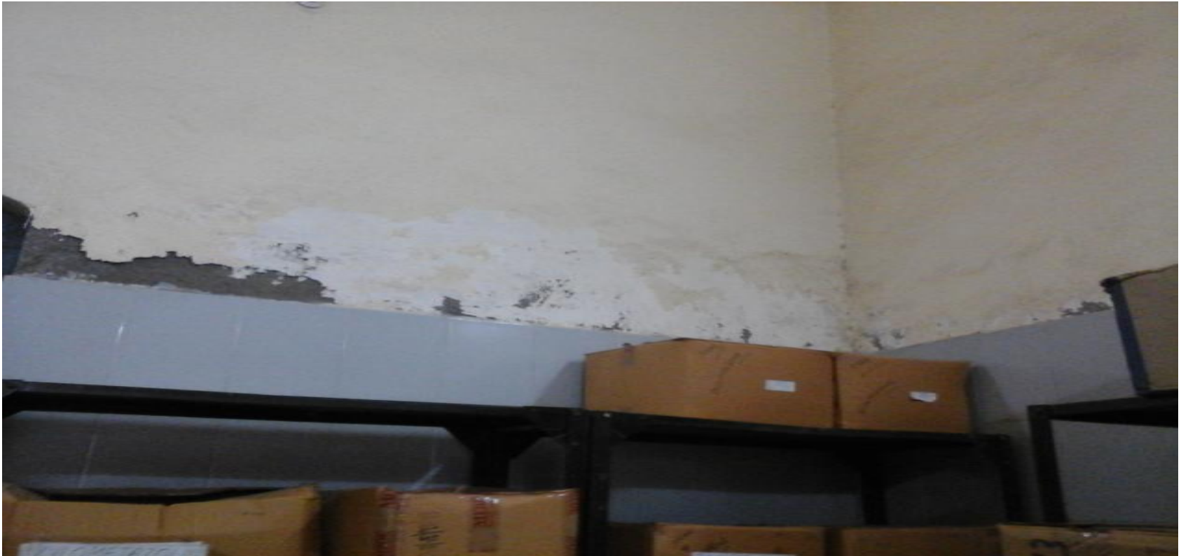
Seepage in main store
