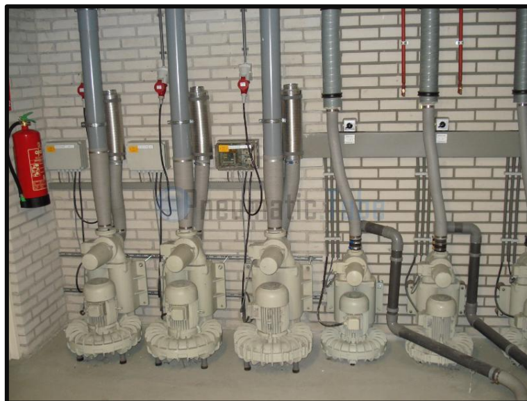
Figure 1.4- Blowers of Pneumatic Tubes
