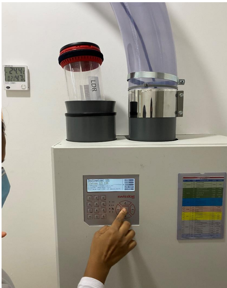
Figure 10- Pneumatic Tube System
