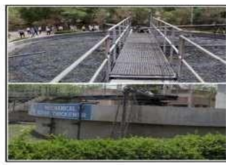
Fig.3.4 Sludge thickener of STP
