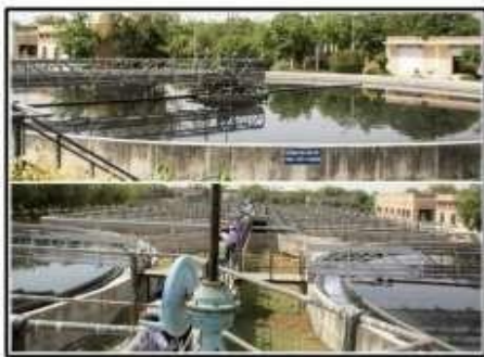
Fig. 3.3 Primary and Secondary Clarifier
