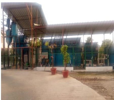
Sewage Treatment Plant
