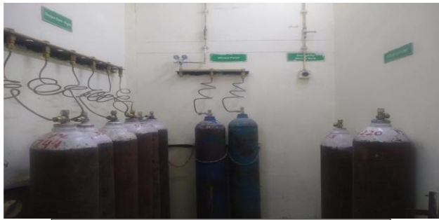
Gas Plant Room
