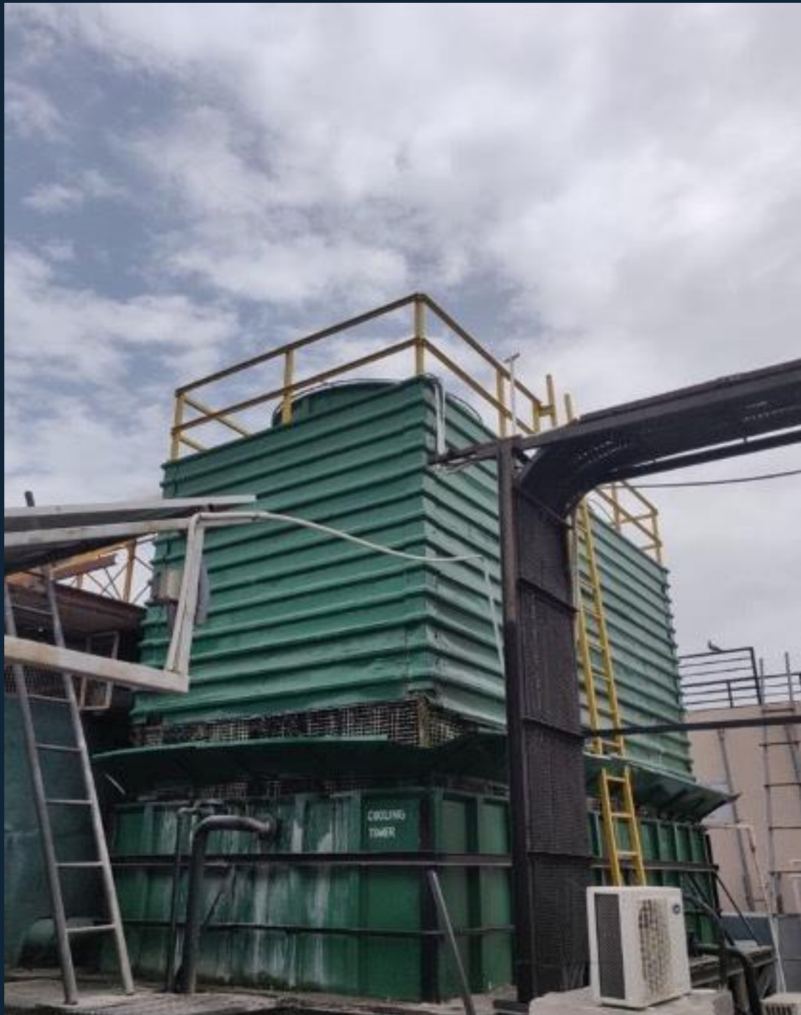
Fig 7: Chiller Plant at BMCHRC
