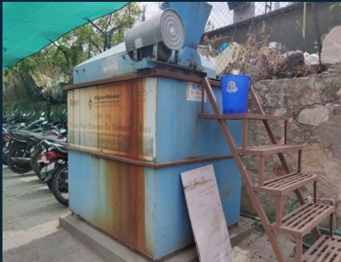
Fig 1: Bio Methanation Plant at BMCHRC
