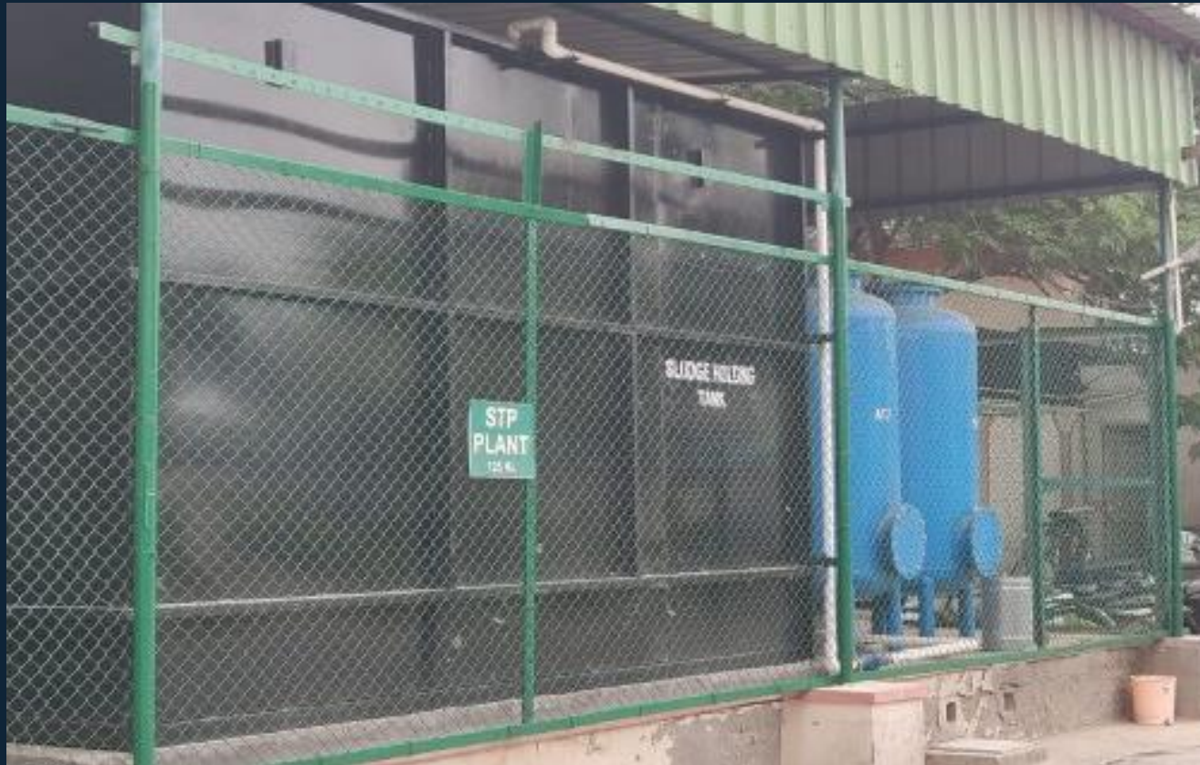
Fig 3: Sewage Treatment Plant at BMCHRC
