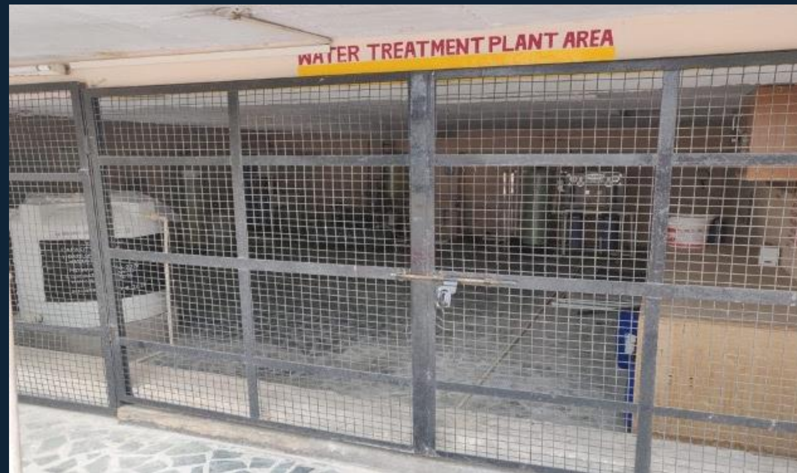
Fig 18: Water Treatment Plant at BMCHRC
