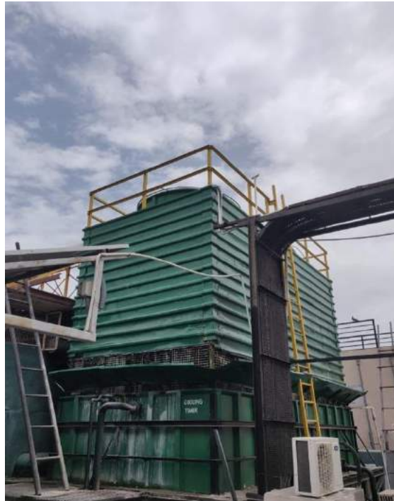
Fig 9: Chiller Plant at BMCHRC
