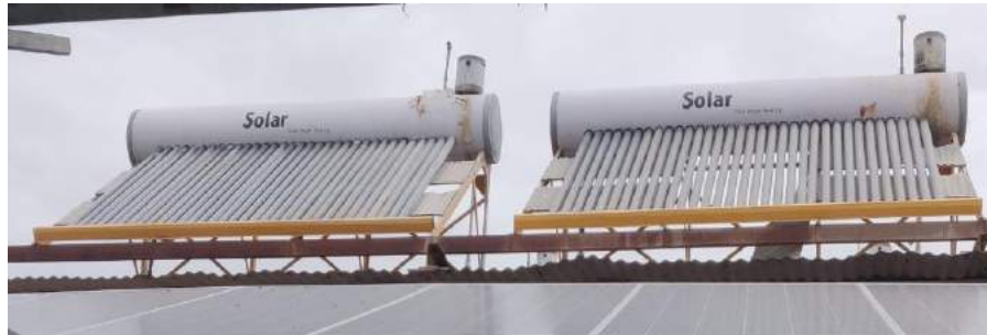
Fig 10: Hot Water Solar Panel at BMCHRC
