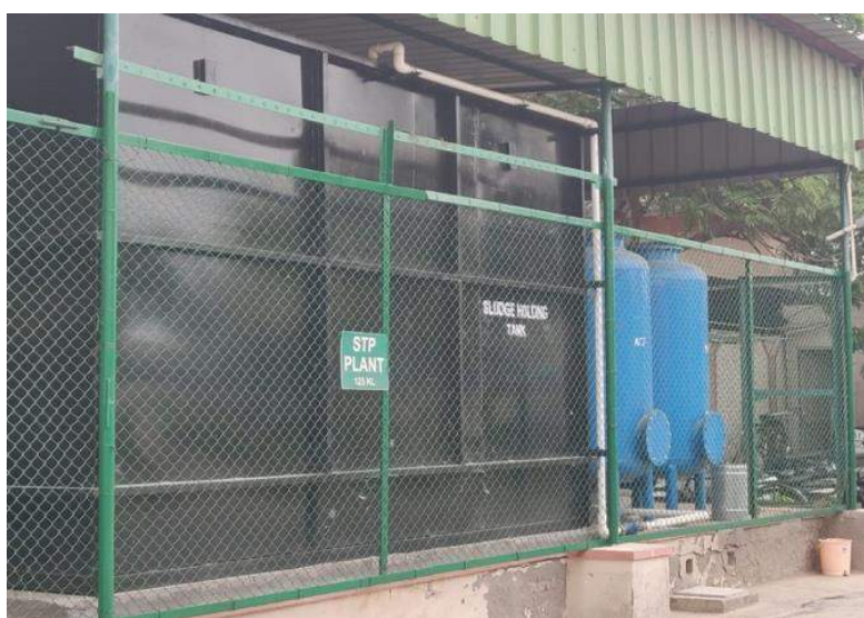
Fig 5: Sewage Treatment Plant at BMCHRC
