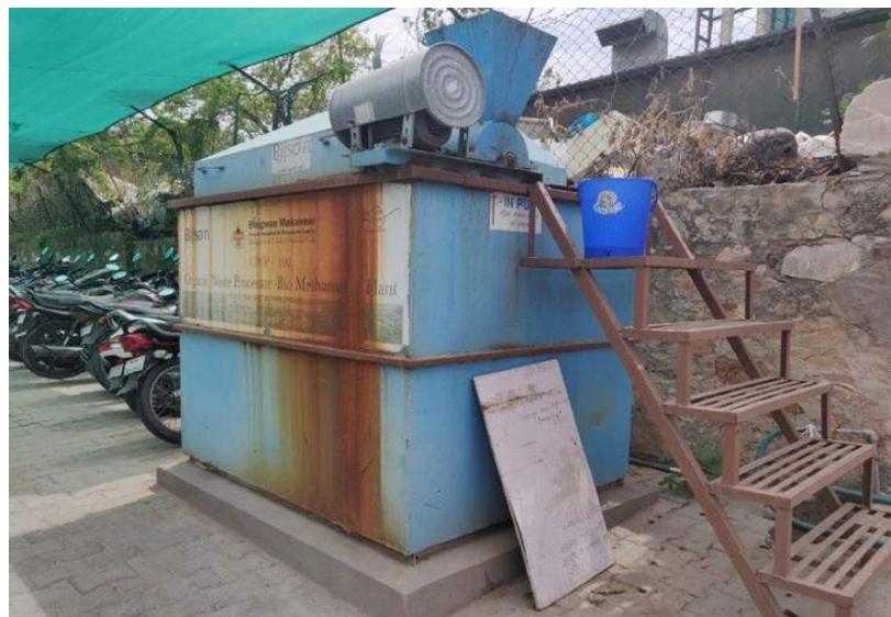
Fig 3: Bio Methanation Plant at BMCHRC
