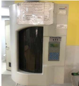
Figure 1.5- Pneumatic Telecom Monitor station
