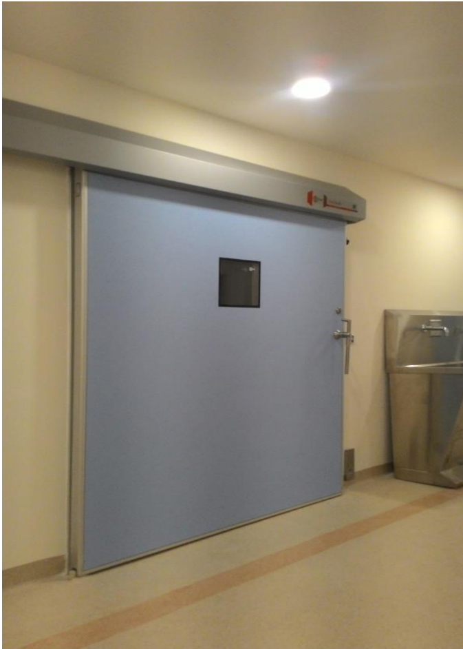
Fig.no.7.4 sensor controlled sliding door
