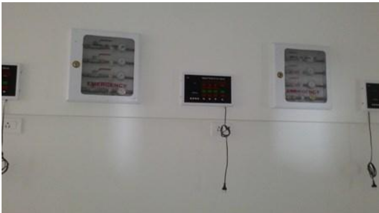
Fig.no.7.19emergency gas alarm
