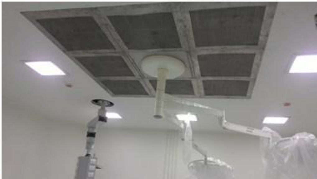
Fig.no.7.11 Hepa filters in CARE OT.
