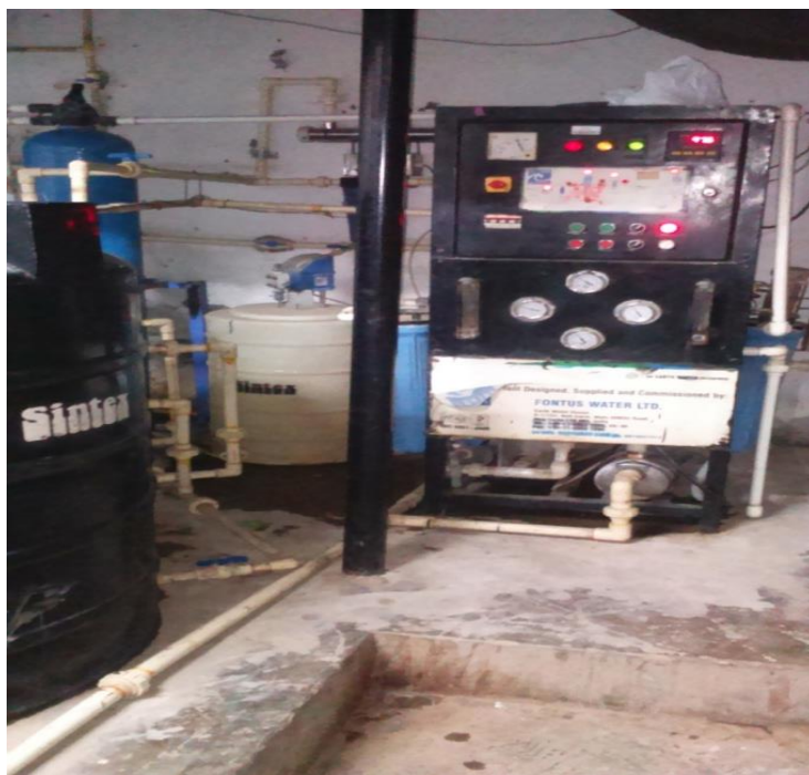
Fig: 1.6.4: RO water treatment plan for dialysis in Paras hospital
