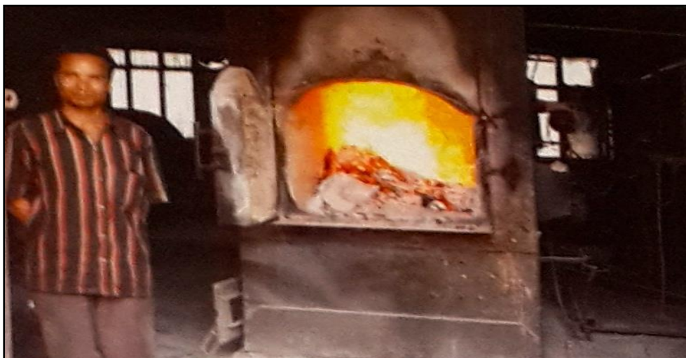
Image of the bio-medical waste department (incinerator) of the hospital
