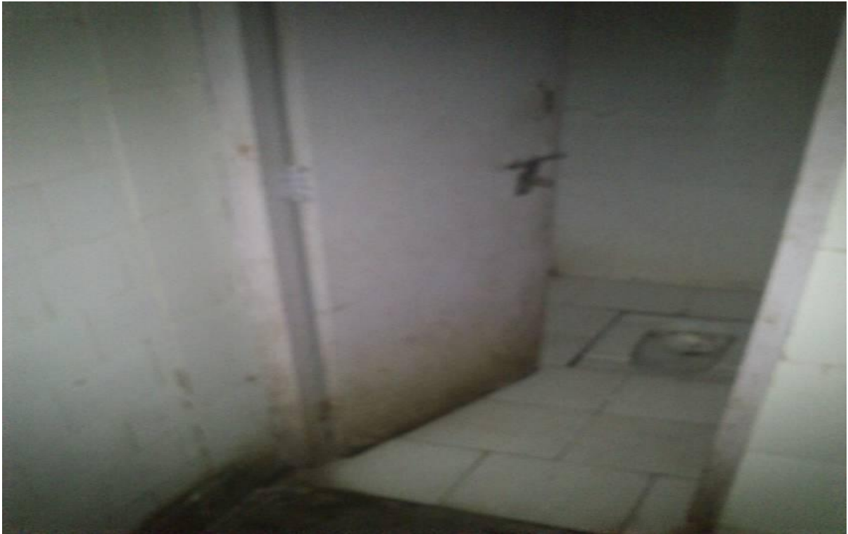
Figure 1: FBNC & Labour room connected with functional toilet
