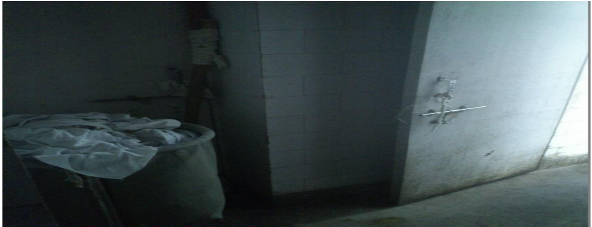
Figure 5: No Utility Room
