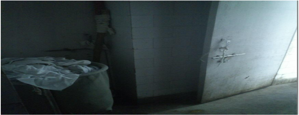
Figure 5: No Utility Room
