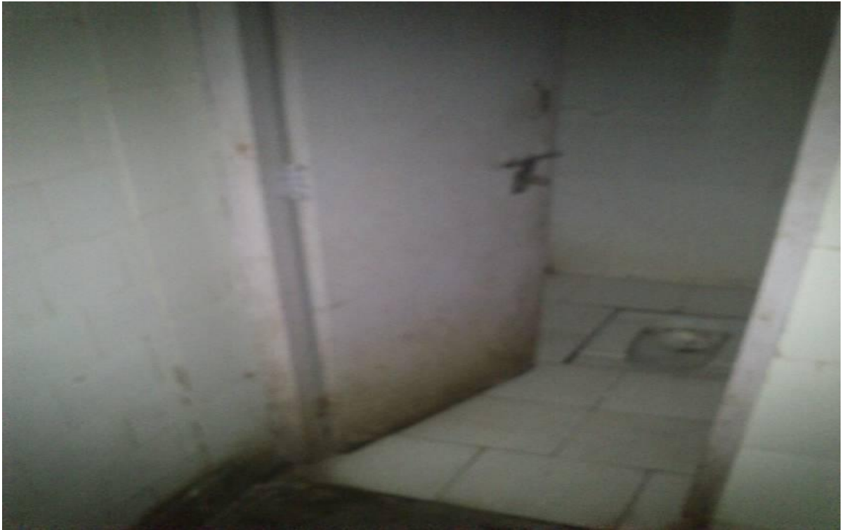
Figure 1: FBNC & Labour room connected with functional toilet
