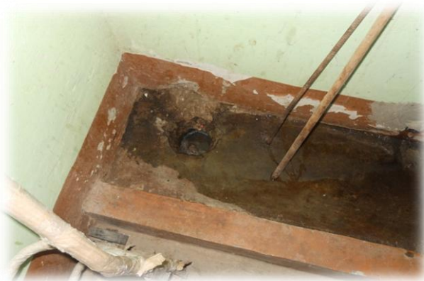
Picture: Showing the condition a labor room in PHC Kakapora.
