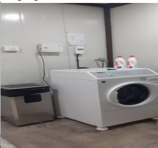
Fig- Disinfectant Room
