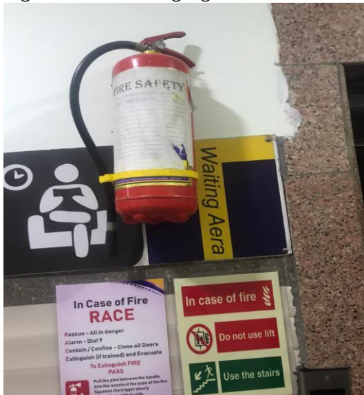
Fig Fire extinguisher with RACE-PASS
