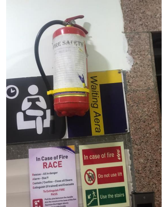
Fig-Fire extinguisher with RACE-PASS
